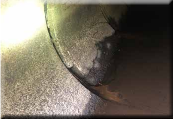
Misaligned joint with voids
