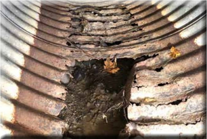
Invert rusting and voids underneath
