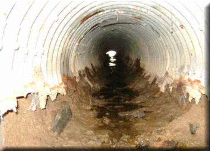
Complete loss of pipe bottom/invert
