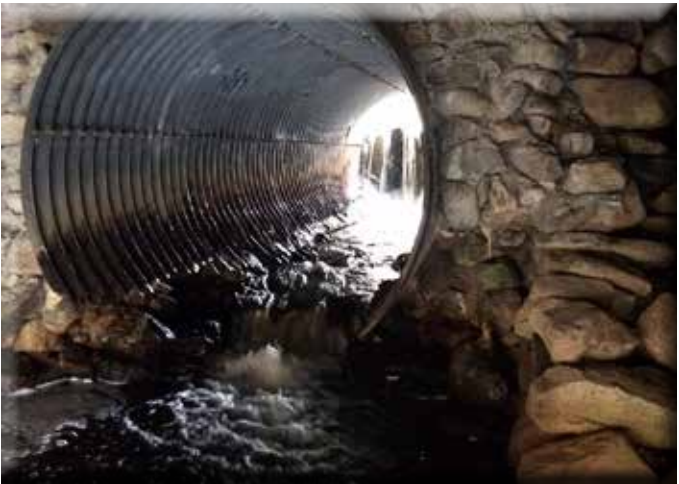
Loss of bottom from pipe exit
