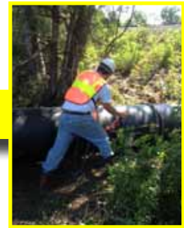
Using chains and pressure from the excavator, the two pieces of pipe are 'snapped' together. The process is repeated until connected sections of Snap-Tite are pushed through the entire length of the culvert.
