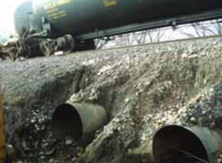
An example of two side-by-side, typical deteriorated culverts close to failure, potentially leading to track collapse and danger to the railroad.
