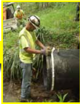
A gasket is installed on the next piece of pipe, assuring a watertight seal when connected.
