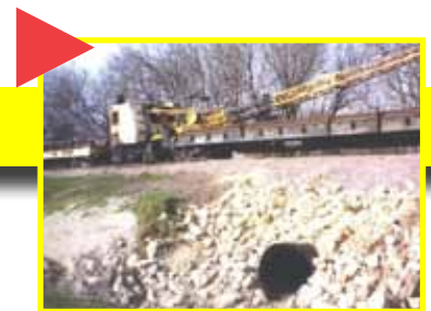
The totally rehabbed Snap-Tite culvert. Nearly all the work was completed off-track in the culvert itself.
