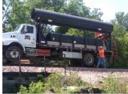
After the culvert is excavated and prepared for Snap-Tite rehab, companies often high rail to deliver the pipe to the project site.
