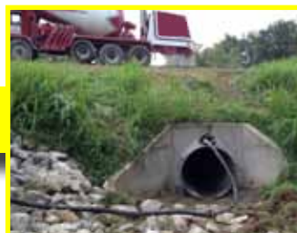
The grout is pumped into the entire length of the pipe, filling in the annular space between the new and host pipe, and the voids outside of the host pipe.
