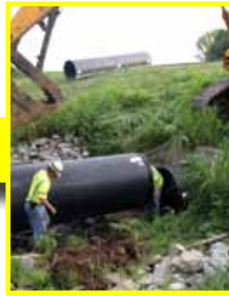
The second piece of pipe is lowered into position, and lined up with the first piece.
