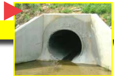
The totally rehabbed Snap-Tite® culvert. Nearly all the work was completed off-road in the culvert itself.
