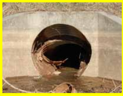
A typical deteriorated culvert in failure mode, proving a danger to the integrity of the flood control structure.
