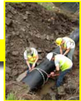
Using chains and come-a-longs, the two pieces of pipe are 'snapped' together. The process is repeated until connected sections of Snap-Tite® are pushed through the entire length of the culvert.
