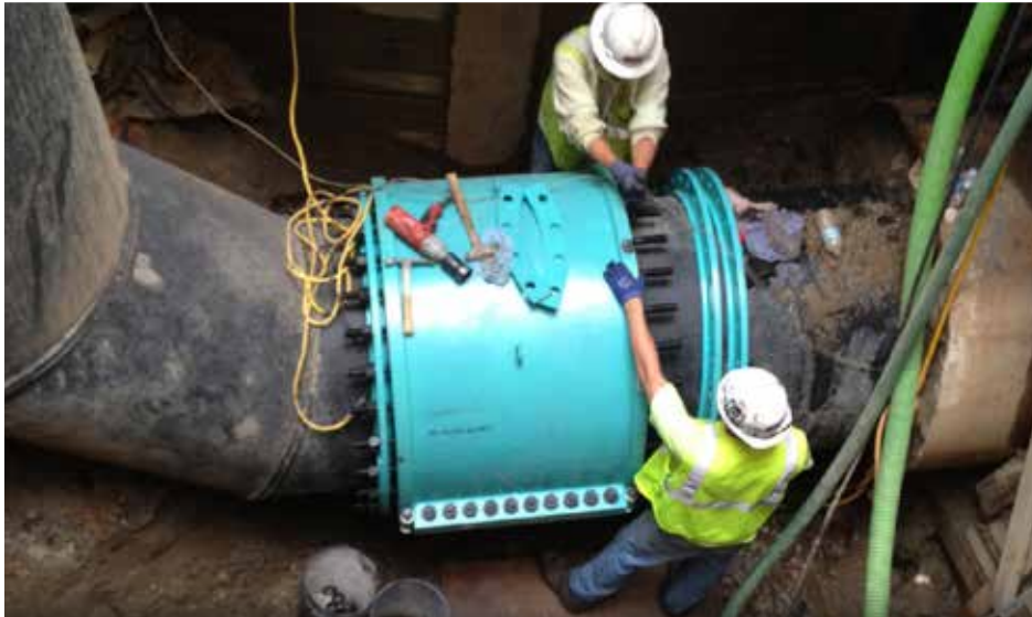
Ohio State University Chilled Water Line
