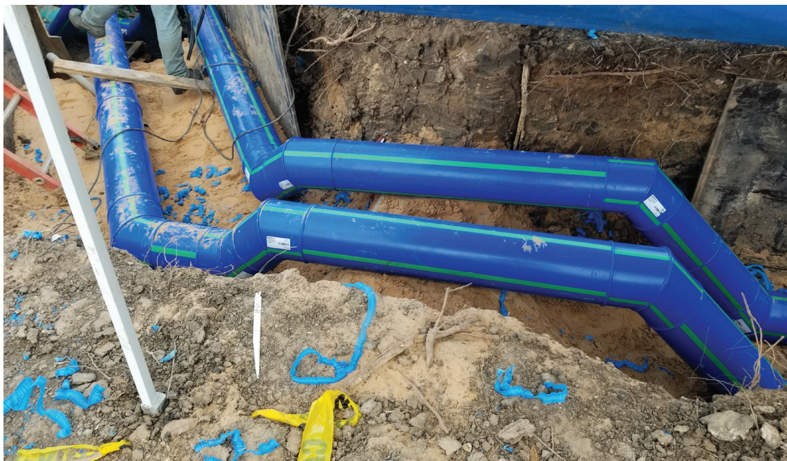
The sections of the Aquatherm pipe that were direct-buried at San Jacinto College South did not require insulation and will last for decades despite the highly expansive soil conditions.
