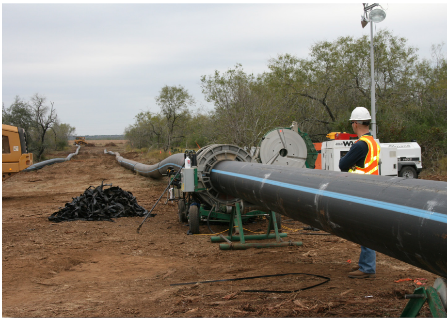
ISCO representative viewing a string of 24-inch DR 9 pipe on the SAWS project
