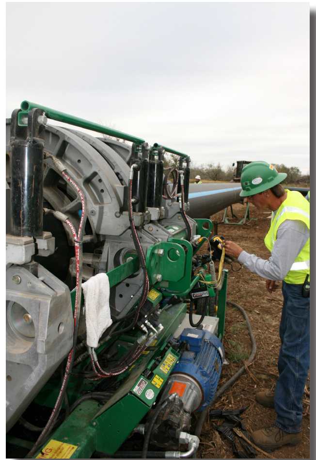
Quality control was a top priority for SAWS and ISCO. An ISCO field fusion technician logs information using a McElroy DataLogger™. The pipe is 24-inch DR 9.
