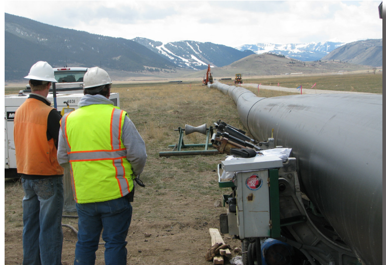
Large-diameter HDPE pipe is fused on site. Photo courtesy of Westwood Curtis.
