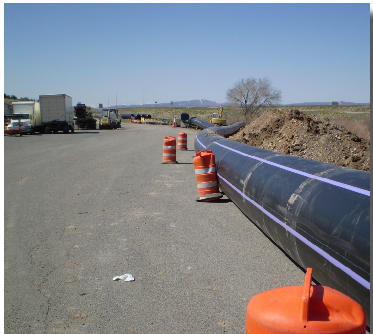
The fused pipe will replace an open ditch irrigation canal with a piped canal. The pipe seen here awaits installation.
