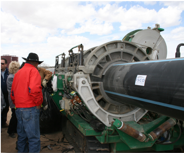
A demonstration of the HDPE pipe fusion using a McElroy fusion machine.
