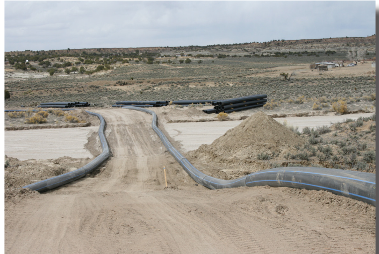
HDPE pipe awaiting installation. Most pipe will be fused prior to installation.
