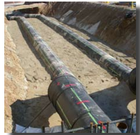
The 36-inch ESW lines were backfilled using flowable fill poured in lifts.
