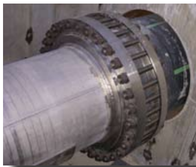
ESW: Flanged connection between the 36-inch HDPE pipe and stainless steel pipe.
